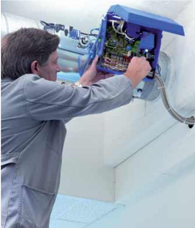
Commissioning of EASYLAB
